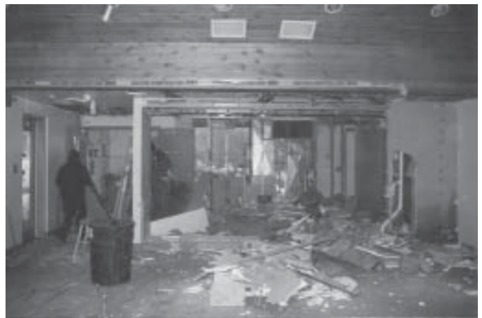
Here is the same view as construction got underway. Hopefully it will look a little better than this at the grand re-opening on May 8. Be sure to stop by and see for yourself.
